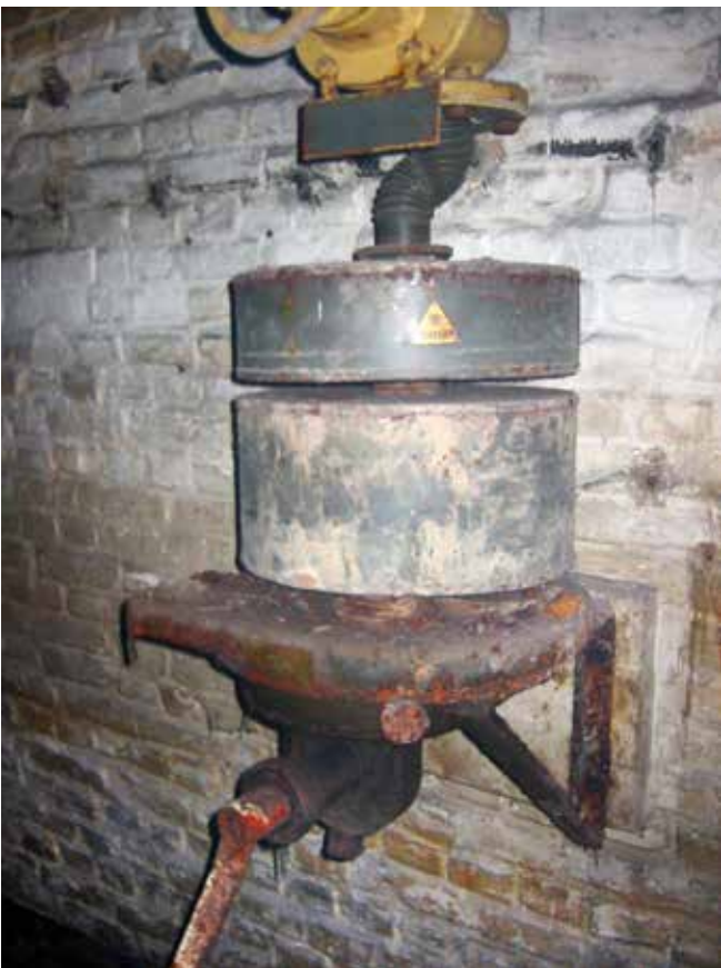
A Draeger ventilation unit with manual crank (in the event of a power failure) halfway up the wall. Photo Andreas Steinhoff reproduced from Wikimedia Commons under creative commons licence
